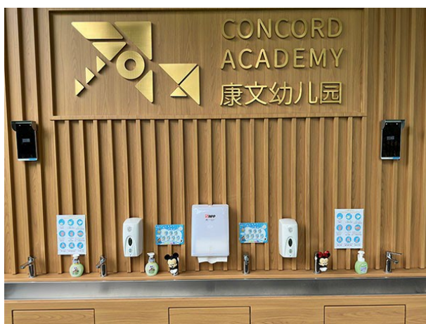
Hand soap installations in a kindergarten
