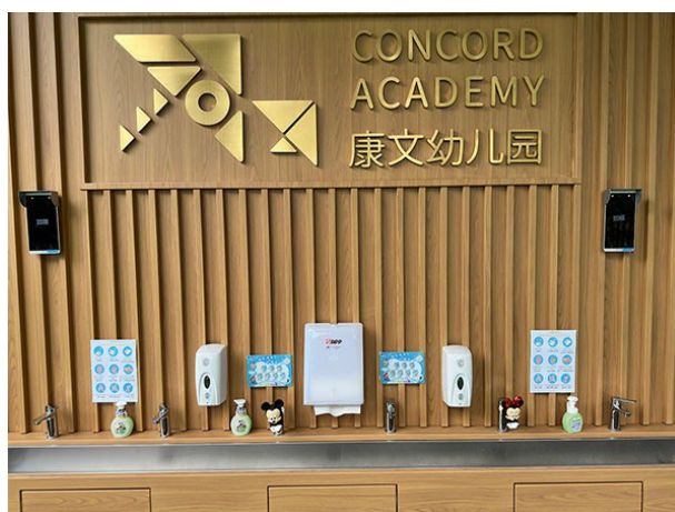
Hand soap installations in a kindergarten
