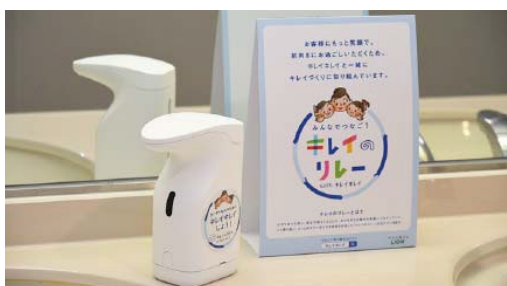
Installation of automatic soap dispensers in toilets at Kakogawa City Hall in 2021 (Kirei Relay Project)
